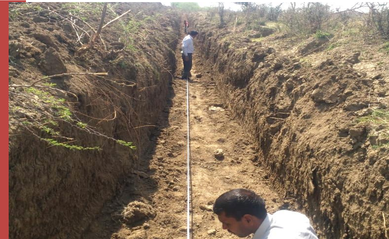
Cattle Protection Trench
